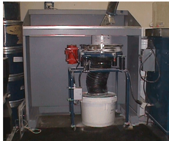
Front view of BOS table showing sifter under the BOS table. (Air handler also shown on the right side of the photo below.)
