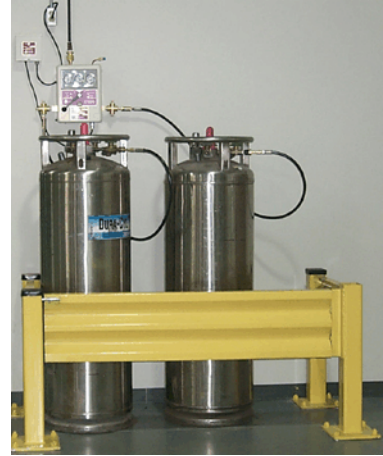
Nitrogen dewars with auto-switching manifold
